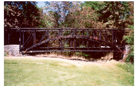
Bridge after it was destroyed by arson
